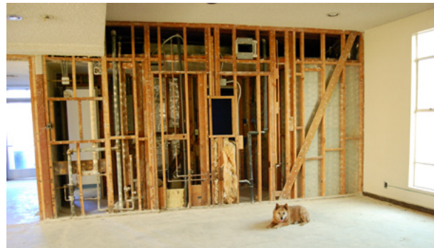
This Chapel wall needs to be upgraded to a 1 hour fire wall because the area on the other side of this wall is a bedroom.
