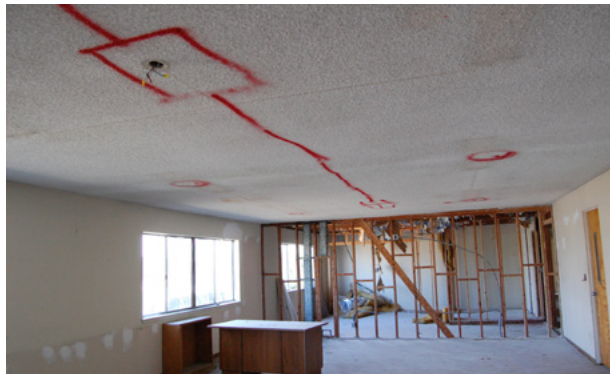
The ceiling in the future 3rd floor community room will be removed for insulation and to install new light fixtures and social communication wiring.
