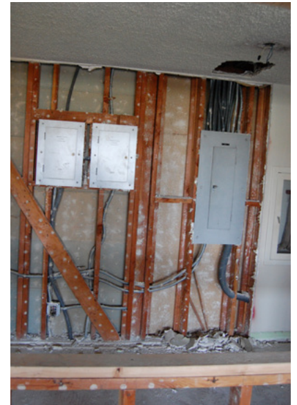
Interior walls are opened for new electrical wiring or panel, and to remove old plumbing and conduit pipes.
